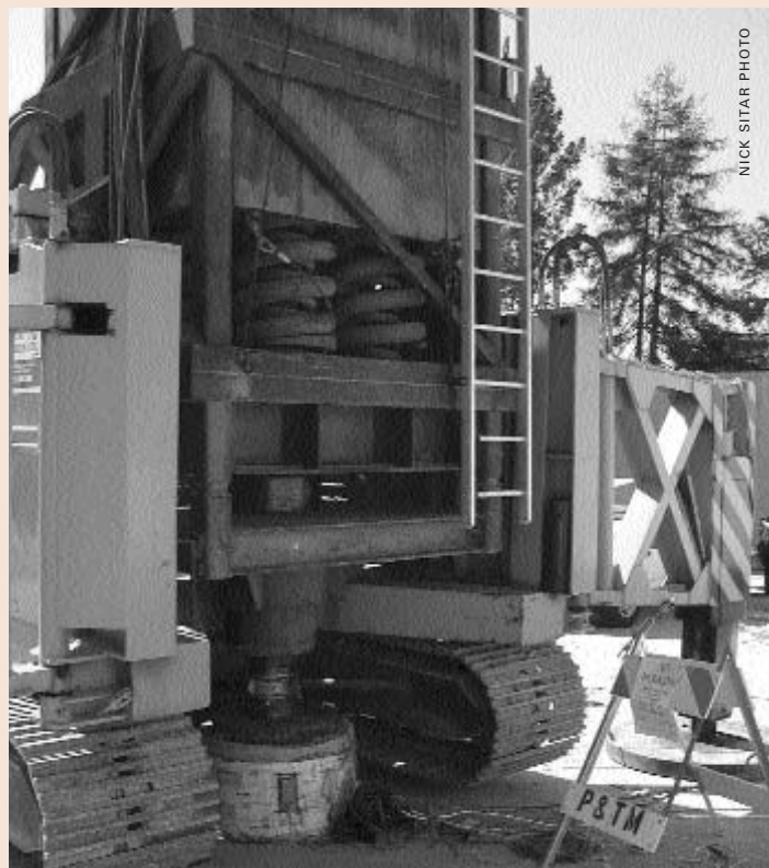
Berkeley architects, engineers, and administrators teamed up last fall to test the seismic strength of foundation piers at a campus construction site. Using an innovative dynamic testing device, above, engineers collected and analyzed data that will lead to more effective retrofitting and lower construction costs.
