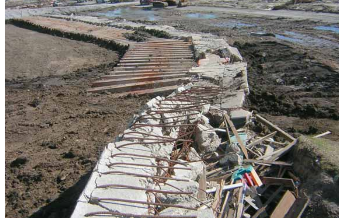
LEFT: Damaged levee floodwall adjacent to a major breach along the Industrial Harbor Navigation Channel in New Orleans's devastated Lower 9th Ward.
