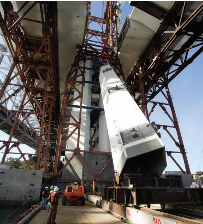
SUPPORT STRUCTURE: A segment of the tower is hoisted into place. SAS designs pose challenging construction problems. "If the deck is needed to hold the cable and the cable is needed to hold the deck, it's like the chicken and the egg. Which one do you build first?" Nader explains. The answer: a steel truss bridge—or falsework—to support the permanent bridge. Seen here underneath the roadbed, the falsework will be taken down after the cable is installed and bears the bridge load.
